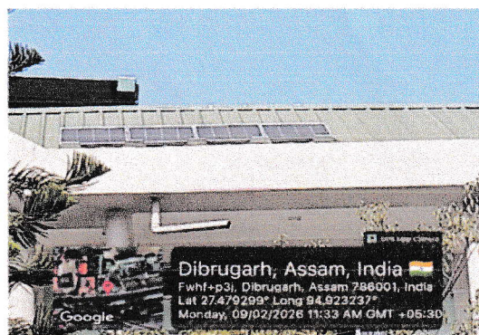
Rooftop solar panels in the main campus
