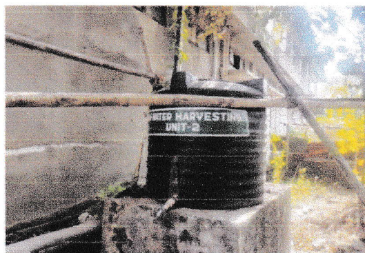
Rain water harvesting unit in the Khaliamaricampus
